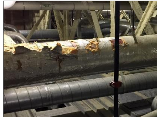
Asbestos-containing brown/red mastic on ducts, Interstitial.
