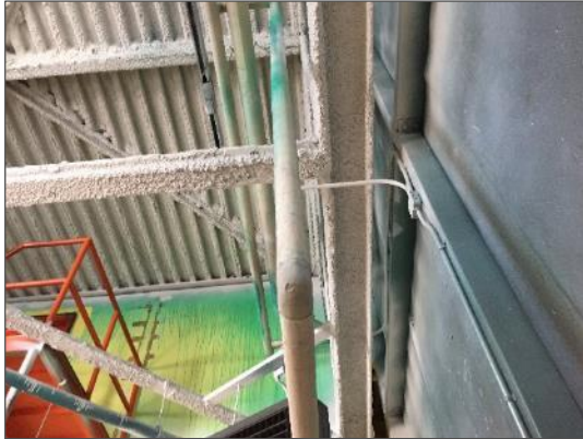
Asbestos-containing parging cement on pipe fitting, Level 6 Mechanical Penthouse.
