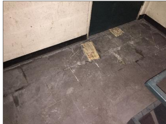
Photo 4 - Damaged asbestos-containing vinyl floor tiles, Stairwell 42 between Level 1 and Level MM.
