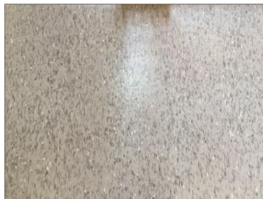
Asbestos-containing vinyl sheet floor, brown square pattern, Level 3 Room 3U35.
