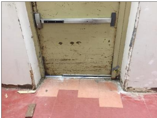
Photo 5 - Damaged asbestos-containing drywall joint compound and debris, Level 1 Exit Corridor at Shaft 88.
