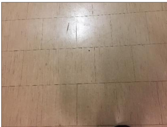
Asbestos-containing 12" x 12" vinyl floor tiles, beige with brown lines.
