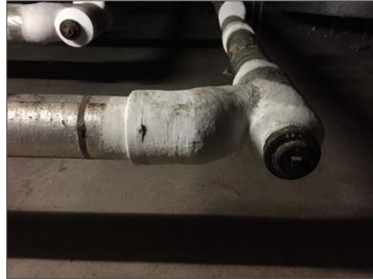
Asbestos-containing parging cement on pipe fittings, MM Level.
