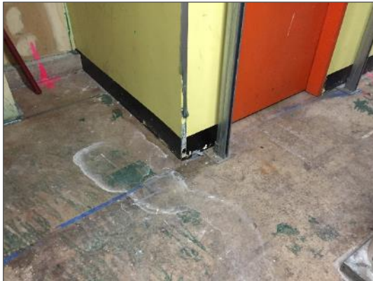
Photo 9 - Damaged asbestos-containing drywall joint compound and debris, Level 6 near Shaft 52.
