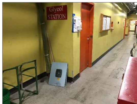
Photo 8 - Damaged asbestos-containing drywall joint compound, Level 6 near Glycol Station.
