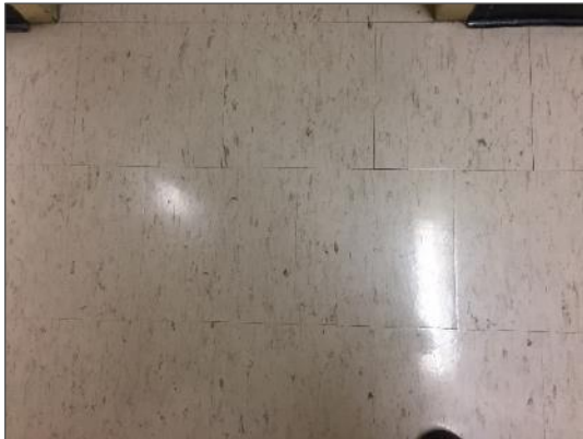
Asbestos-containing 12" x 12" vinyl floor tiles, white with brown flecks.
