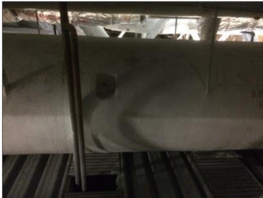
Asbestos-containing insulation on exhaust ducting, Interstitial.
