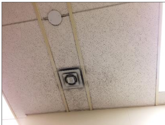
Asbestos-containing lay-in ceiling tiles, large and small pinhole pattern, Level 1 Room 1J8.
