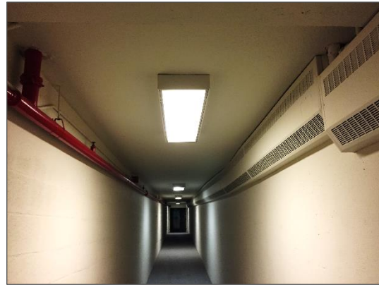
Asbestos-containing texture finish, Corridor from Elevator 22 to Parking Garage.
