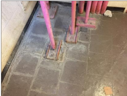
Photo 3 - Damaged asbestos-containing vinyl floor tiles, Stairwell 56 between Level 1 and Level MM.
