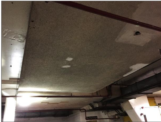
Asbestos-containing texture finish, Southeast corner of Yellow Parking Garage.
