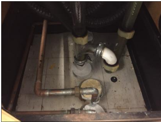
Asbestos-containing parging cement firestopping is present at pipe penetrations below laboratory sinks.
