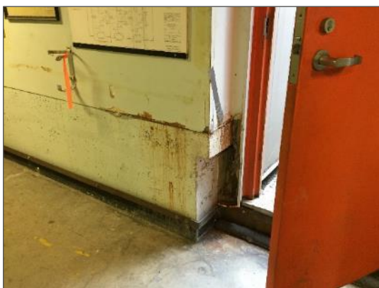
Photo 7 - Damaged asbestos-containing drywall joint compound, Level 6 near Elevator Room 23.
