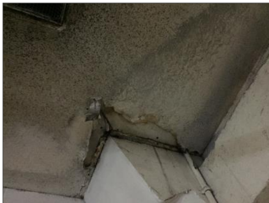
Photo 1 - Damaged asbestos-containing texture finish on bulkhead, Southeast corner of Yellow Parking.
