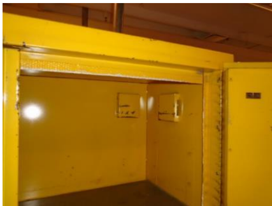
Asbestos-containing textile gaskets on typical flammable storage cabinet, Level 3 Laboratory.
