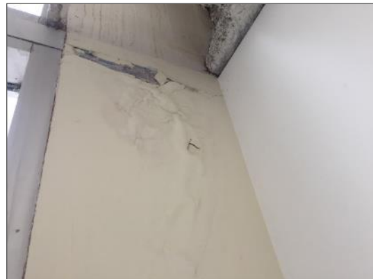
Photo 6 - Damaged asbestos-containing drywall joint compound, Level 3 near Courtyard 2 and Shaft 74.
