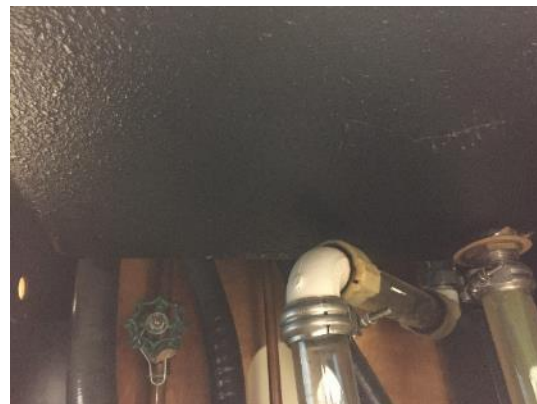
Asbestos-containing black mastic sink undercoating, Level 4 Laboratory.
