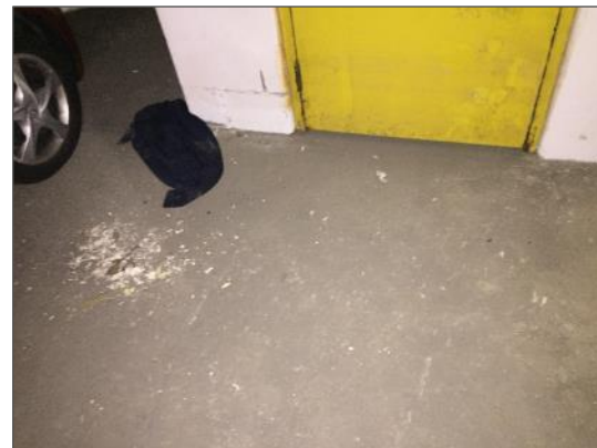
Photo 2 - Asbestos-containing texture finish debris, Southeast corner of Yellow Parking.
